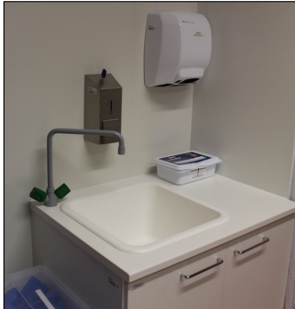
Figure 9: Building A, Entrance Filter (A 1.05) – Area dedicated for cleaning
