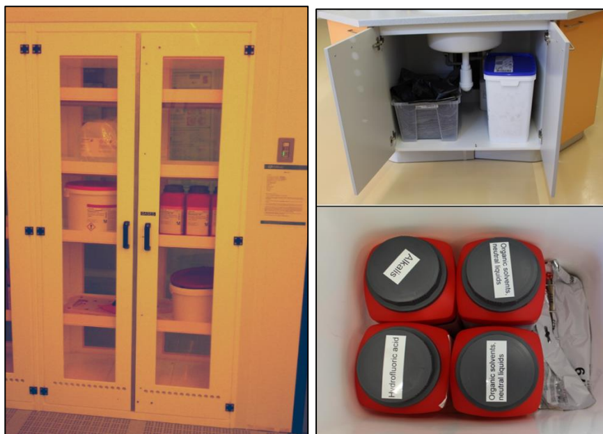
Figure 28: Spill kit in Chemical lab (C 1.31) and in Sample Preparation room 2 (A 1.04)
